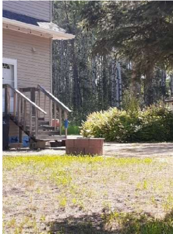
Figure 8: Firepit surrounded by noncombustible material, however, recommend the use of mesh to control sparks.
