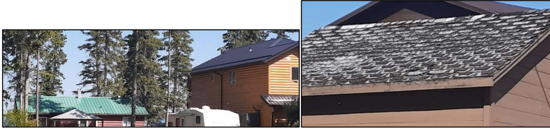
Figure 4: Left picture showing a clean (no leaf litter) metal roofs. Right picture showing asphalt shingles needing replacement.
