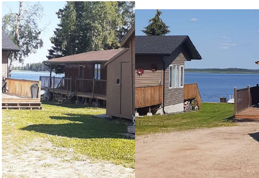
Figure 5: Both pictures showing unskirted decks with dry firewood underneath. Embers could enter and ignite dry leaf litter and firewood in these areas.
