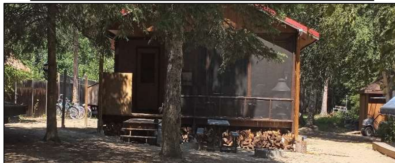
Figure 5: Picture above show foundation that is not skirted. Picture below showing firewood stored underneath deck. Embers could enter and ignite dry leaf litter and firewood in these areas.
