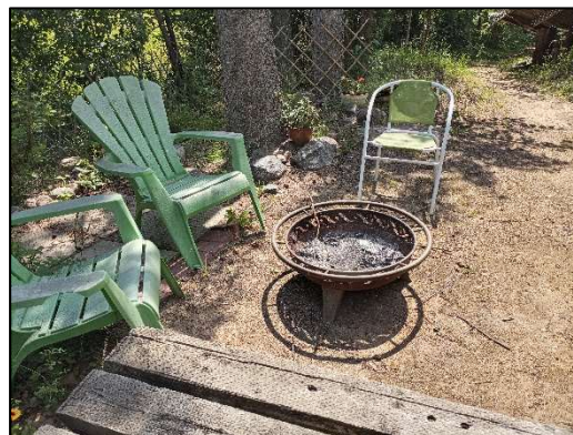
Figure 9: Firepit surrounded by noncombustible material, however, recommend the use of mesh to control sparks.
