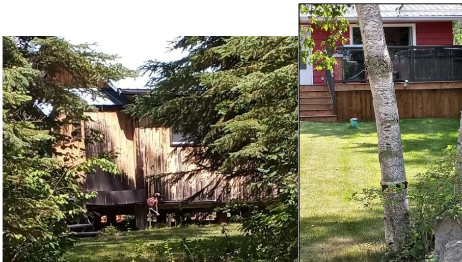
Figure 5: Picture on left show foundation that is not skirted. Picture on right showing skirted in deck area.
