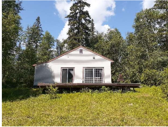
Figure 4: Picture on left show foundation that is not skirted.
