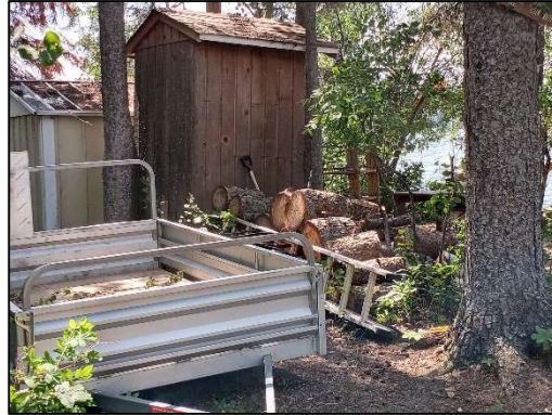
Figure 6: Firewood and other combustibles stored between trees (ladder fuel) and too close to structures provide ignition points and fuel for wildfires.
